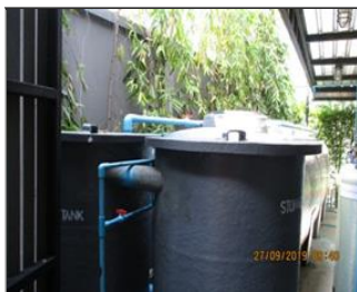
External photo(s) of the production unit(s) WWTP_1.jpg
