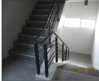
Photo of fire safety equipment secondary exit way.jpg
