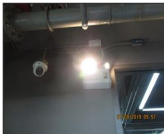
Photo of the dormitories (if applicable) Emergency light.jpg
