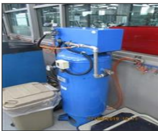
Photo of the inside of the main production hall Air compressor.jpg
