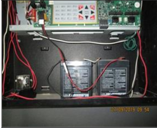
Photo of fire safety equipment Back up fire alarm.jpg
