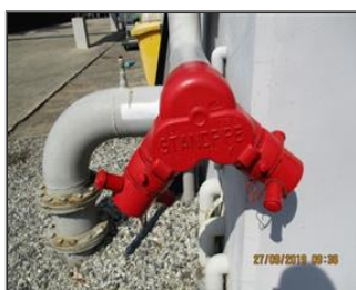
Photo of fire safety equipment Fire hydrant.jpg
