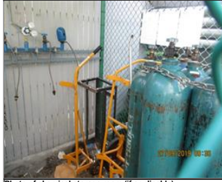
Photo of chemical storage room (if applicable) Gas station_2.jpg
