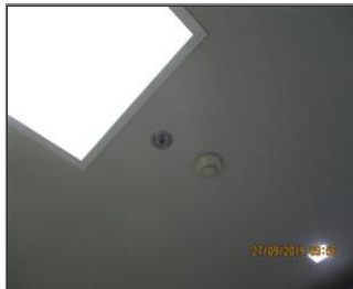
Photo of fire safety equipment Smoke detector and Sprinkle system.jpg
