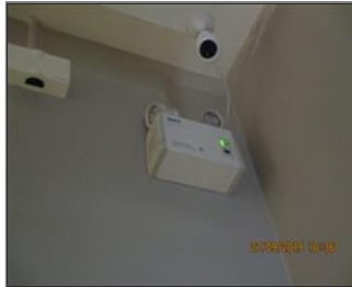
Photo of the dormitories (if applicable) Emergency light box has been installed at owner residence at 7th floor.jpg
