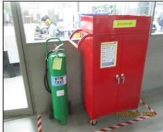
Photo of fire safety equipment Fire extinguisher_2.jpg
