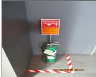
Photo of fire safety equipment Fire extinguisher.jpg
