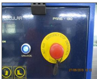
Photo of the inside of the main production hall Emergency stop button.jpg
