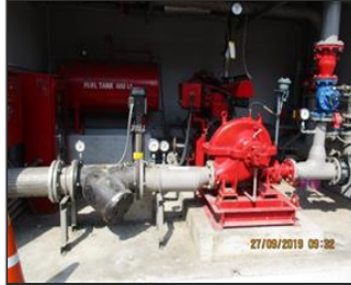
Photo of fire safety equipment Fire pump.jpg
